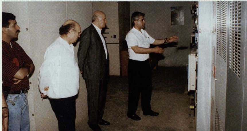
Right, the electrical consultant briefs V.P. Tomey and Physical Plant Director on the project.
